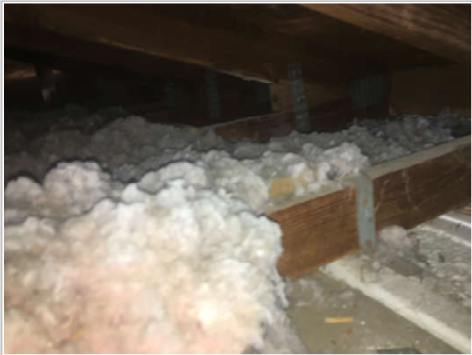
Toe Nail - Not Meeting Nail Requirements
