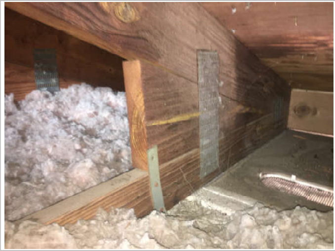
Toe Nail - Not Meeting Nail Requirements
